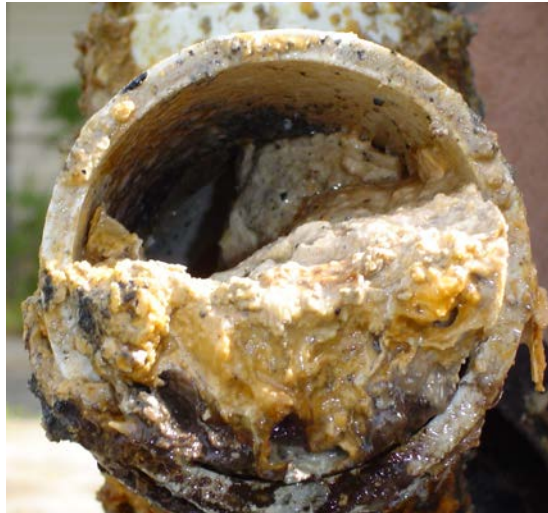
Photo 1- Fats, grease and food products can solidify and block sewerage pipes
