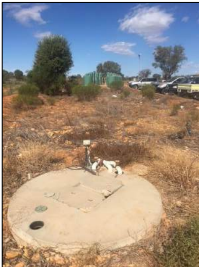
Balance tank. SK-10 units in background
