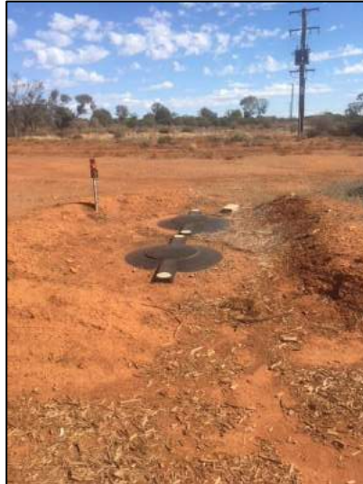
Treatment tank for laundry
